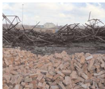
Figure 3. On-site waste management. Masonry rubble visible in the foreground with recyclable steel sections in the background.
