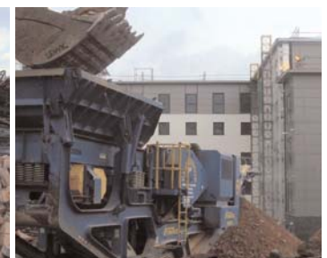
Figure 4. On-site waste concrete crushing plant used to downcycle concrete to secondary uses.
