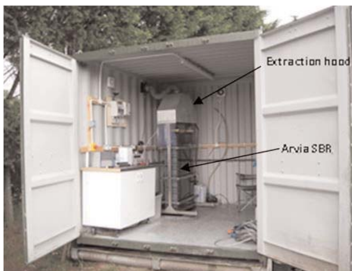
Figure 5: The Arvia™ batch treatment unit (the SBR) – inside the container.
