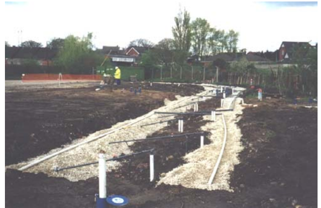
SVE extraction pipework laid horizontally
